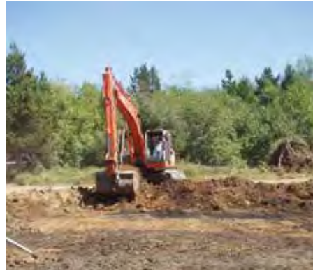
Figure 13. Removing fill from the buried marsh floor. Note the dried grass that was uncovered in the foreground, which confirms the original marsh surface has been uncovered.
