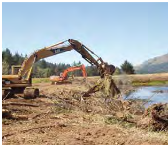
Figure 104. Placing large woody material along the edge of Kingfisher Lake for habitat enhancement.
