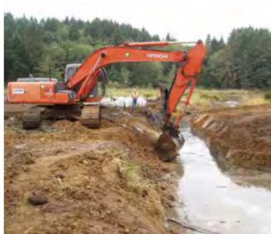
Figure 110. Shaping the stream banks after the culvert and tide gate were removed.
