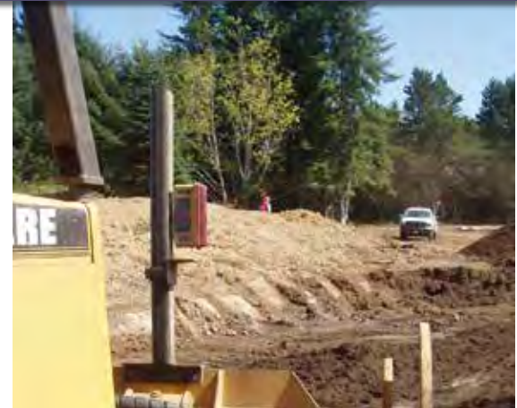
Figure 108. RA laser level eye was mounted on the blade of the bulldozer. This allowed for precise grading in an efficient manner.
