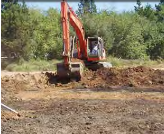
Figure 106. Removing fill from the buried marsh floor. Note the dried grass that was uncovered in the foreground, confirms the original marsh surface has been uncovered.
