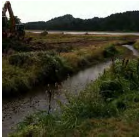
Figure 63. Excavator removing spruce trees and dike, freeing Crowley Creek from the ditch.
