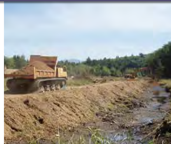
Figure 103. Work in progress on the dike and ditch removal. The tracked dump truck is transporting fill material that will be placed in the ditch.
