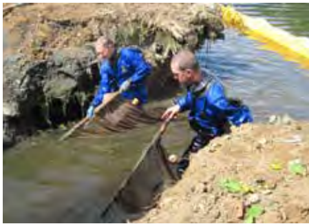
Figure 49. Last pass through waterway with seine net before remaining concrete is removed from tide gate area. Siuslaw National Forest Fisheries Biologists Jason Wilcox and David Skelton pictured.
