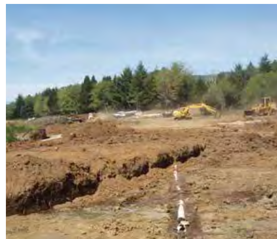
Figure 105. The exposed PVC pipe marks the original marsh elevation. Fill removal is in progress in the background.
