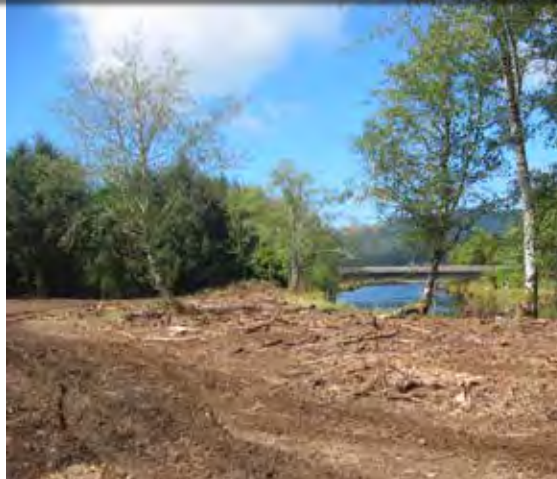
Figure 115. The dike has been removed and reshaped to resemble the natural levee present along other nearby sections of the river. The tide gate house is gone. Woody debris was scattered over the disturbed area.
