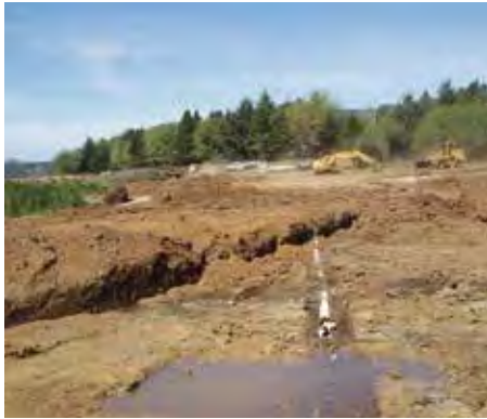
Figure 12. The exposed PVC pipe marks the original marsh elevation. Fill removal is in progress in the background.
