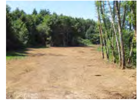
Figure 33. Finished dike removal along Highway 18. The highway is behind the trees on the left.
