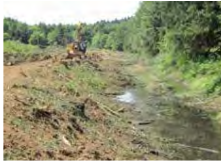
Figure 31. Dike removal and ditch filling in progress along U.S. Highway 101. The highway is behind the trees on the right.
