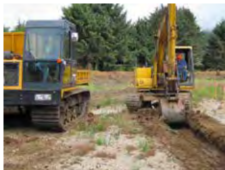
Figure 34. A small meandering stream channel was dug to provide natural drainage to the marsh surface.
