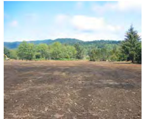
Figure 119. Finished marsh surface after the grading was completed. View to the north.
