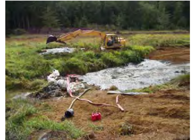
Figure 93. The black goo, or marsh muck, collected behind the coffer dam in the ditch. As the fill was added it pushed the muck toward the end of the ditch. The excavator operator used the bucket to scoop out the muck and place it on the marsh floor behind the excavator.
