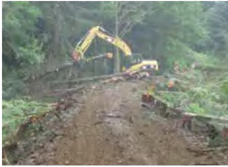
Figure 30. The spruce trees on the dike along Highway 18 have been removed in preparation for leveling the dike.
