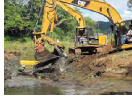
Figure 51. Removing the concrete around the tide gate, August 24, 2011. Jared Richey and Paul Lindsey pictured.
