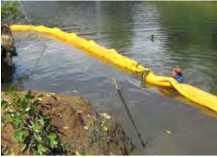
Figure 48. Installing the sediment curtain near the outlet of the tide gate in the Salmon River.
