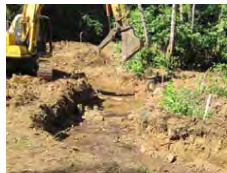
Figure 36. Digging the upstream portion of the new Fraser Creek channel just downstream of Highway 18.
